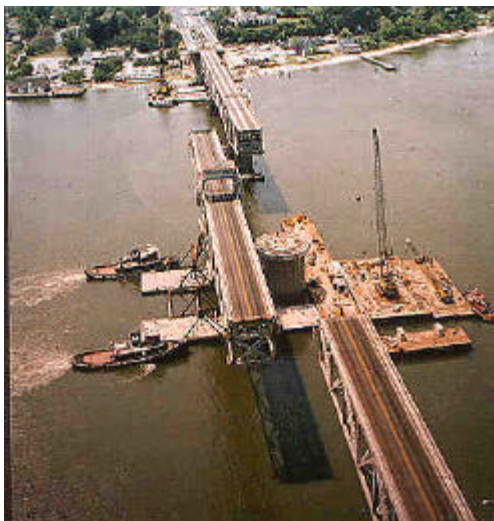
An existing bridge span is removed and floated away for off-site demolition
