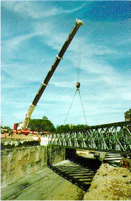
With the help of a crane, a ten-person crew assembled and positioned the two temporary
