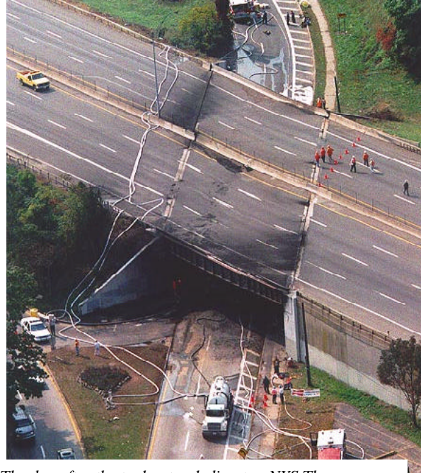
The day after the tanker truck disaster, NYS Thruway authorities and local officials assessed the extent of the damage to the bridge.
