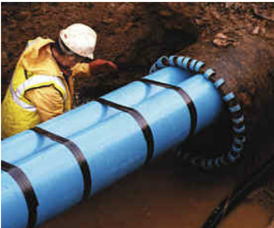
Picture of subline process actually in use, with folded, banded pipe being inserted into older pipe
