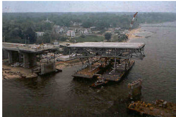
A section of the new bridge span is floated into place. The complete replacement of all bridge sections caused the closure of the bridge for only nine days.
