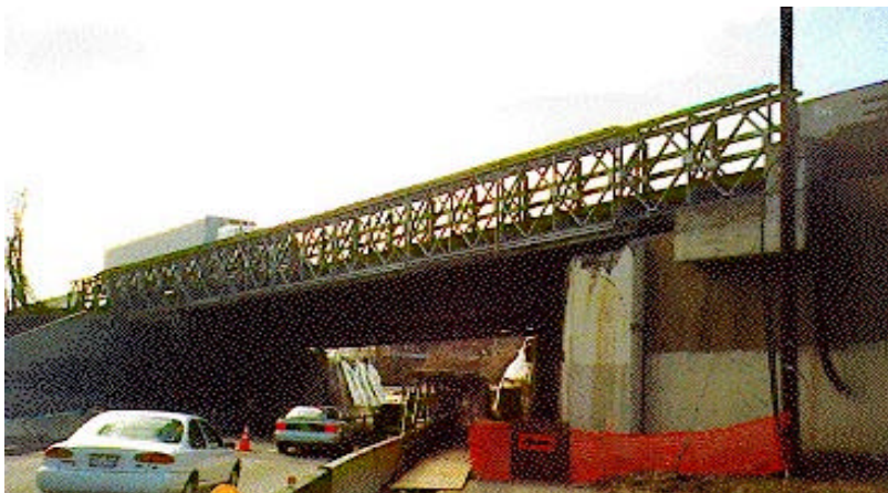
By using temporary bridges, traffic was moving again within eleven days of the accident.
