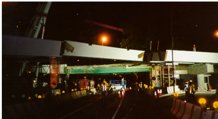
Beam Placement on the 48 th Street Ramp. Completing work at night help to void costly and time consuming congestion during commuting hours.
